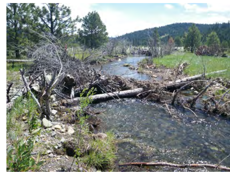
EXAMPLE: INSTALLED CHANNEL SPANNING JAM STRUCTURE
