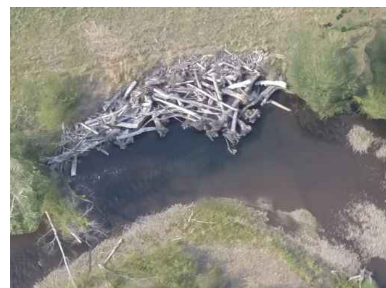
EXAMPLE: INSTALLED BEND JAM STRUCTURE
